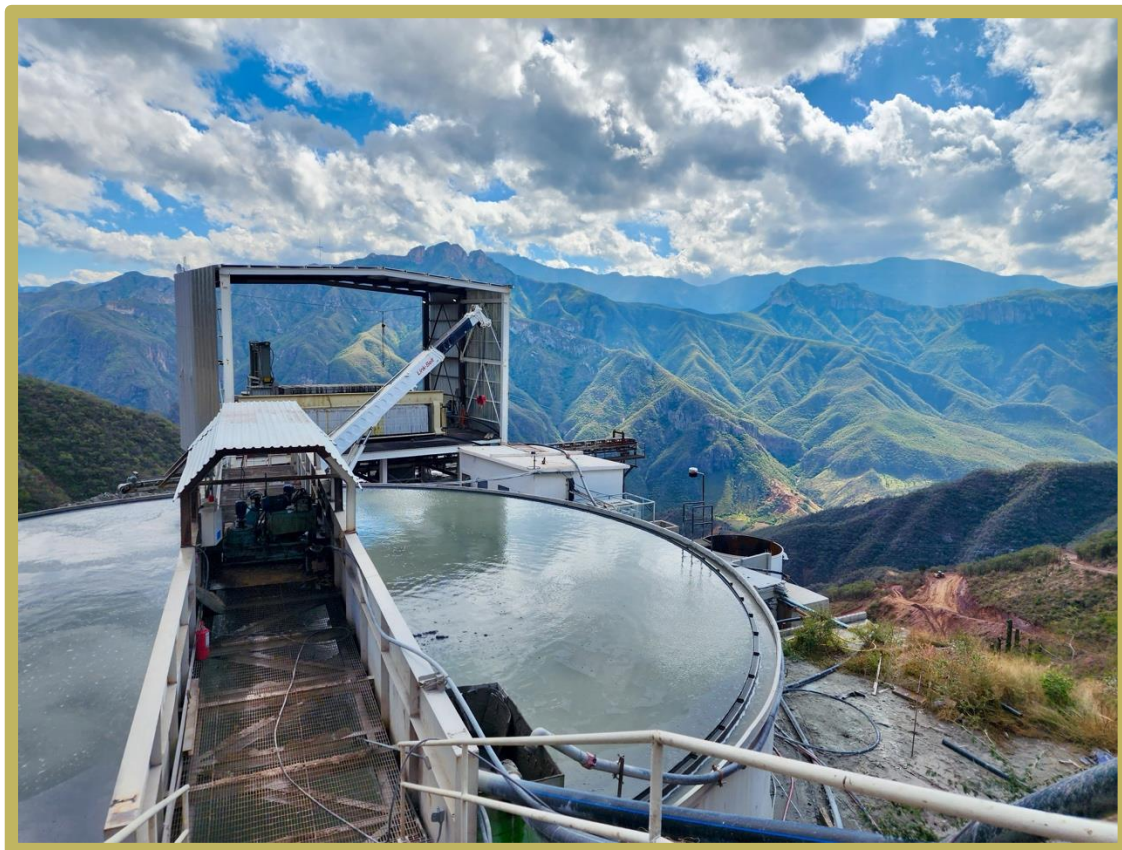
Thickener tank at the Tahuehueto plant
