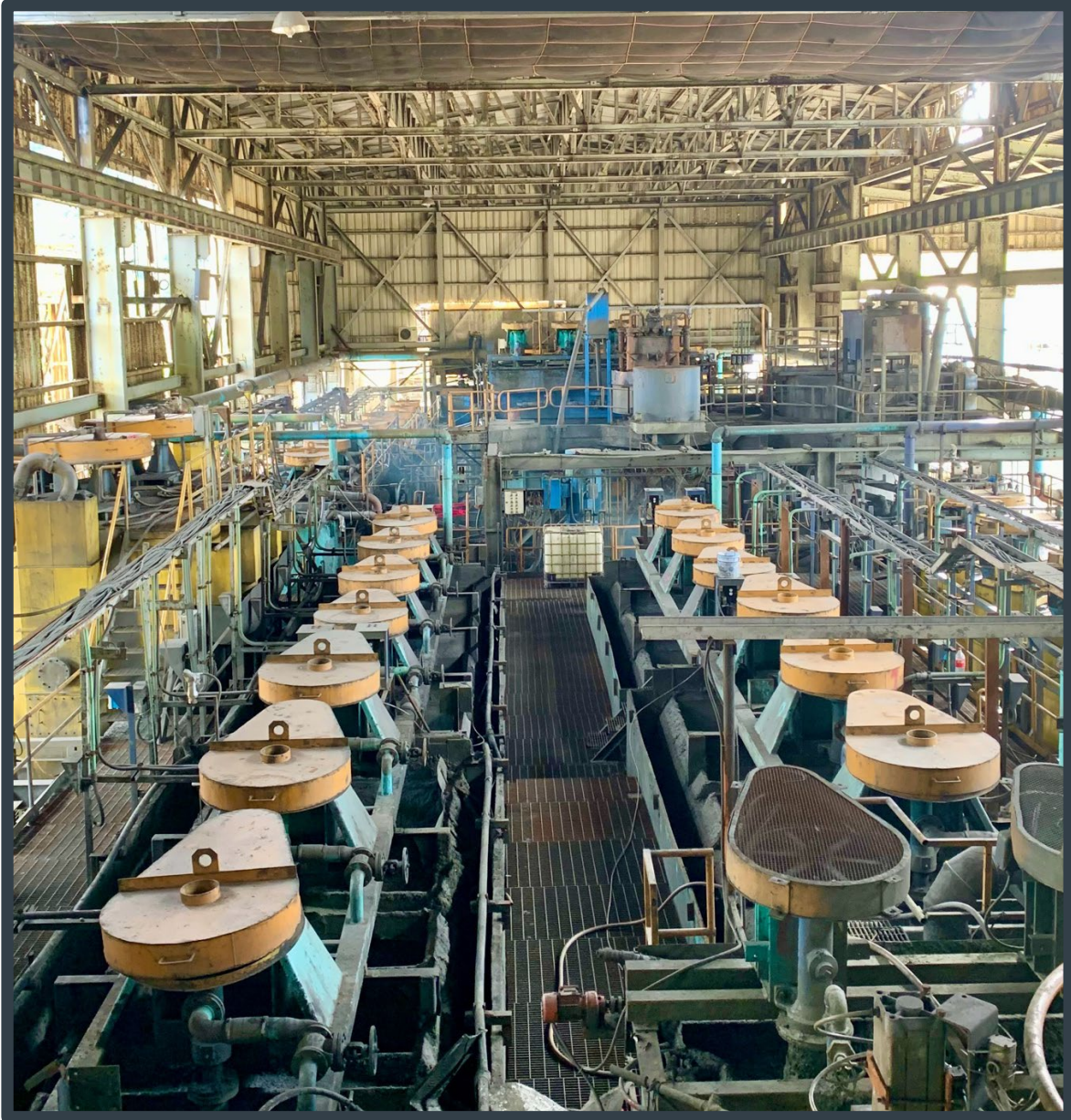
Flotation circuit at Campo Morado
