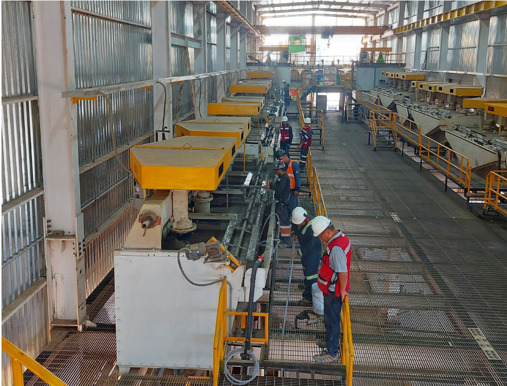
Mill Concentrate Filtration Area
